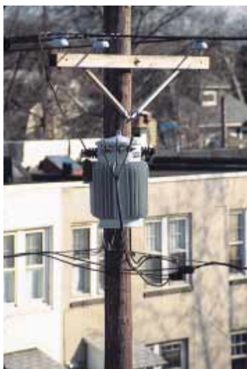
This cylindrical step-down transformer drops the voltage from 4 000 V to 220 V for delivery to a group of residences. (George Semple)
