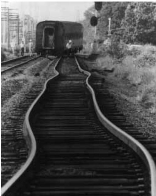
Thermal expansion: The extreme temperature of a July day in Asbury Park, NJ, caused these railroad tracks to buckle and derail the train in the distance. (AP/Wide World Photos)
